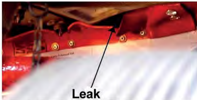
THIS SIGNIFICANT COOLING AIR LEAK , resulting from a wrinkle in a flexible baffle seal, is what caused the T210 CHTs to run so hot.
