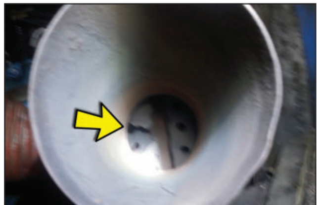
View up the tailpipe. Flame tube is broken, and there's a crack around the base of the tailpipe. The entire muffler assembly will have to be replaced or overhauled.
