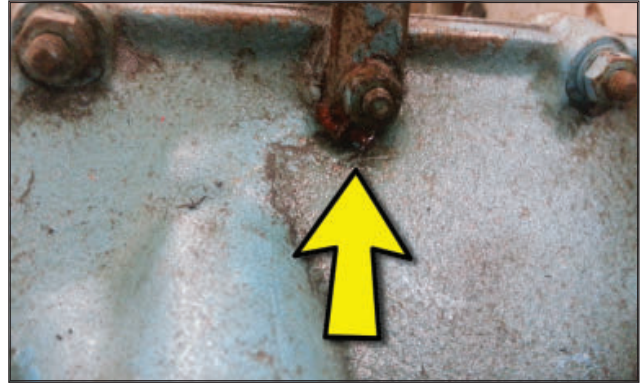
Oil leaking at crankcase top spine bolt. Attempt to stop leak with RTV unsuccessful. Leak will continue until engine is overhauled.
